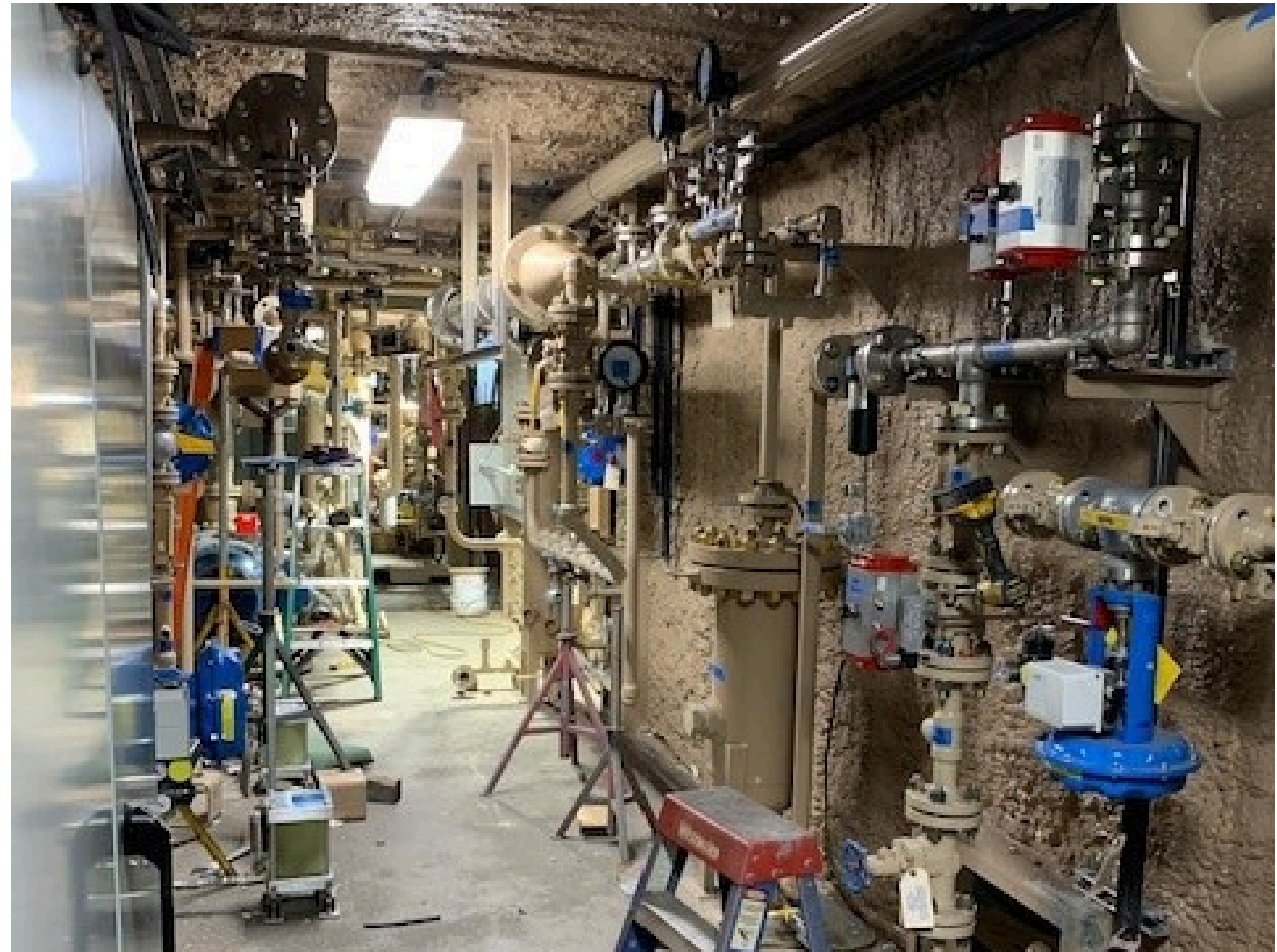
Internal view of 1 of the 4 modular housing units that house the helium processing facility
