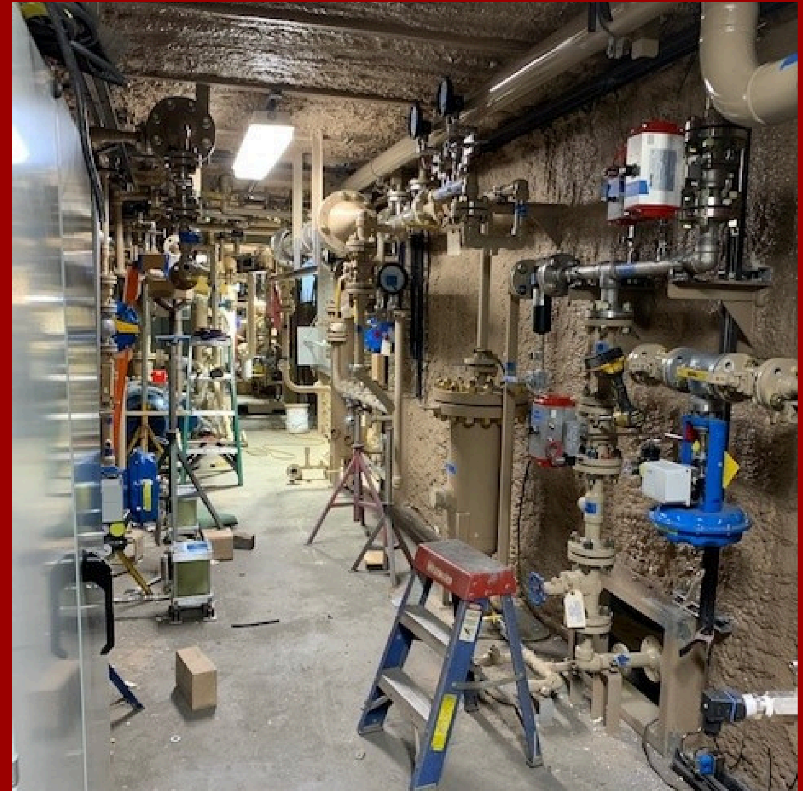
Internal view of 1 of the 4 modular housing units that house the helium processing facility
